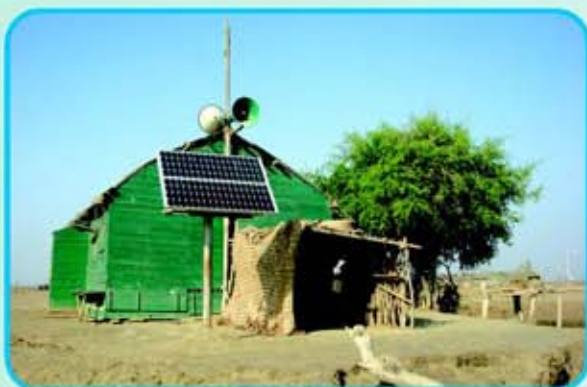
With PCRET's support the Programme has installed solar panels in schools and mosques in the creeks
