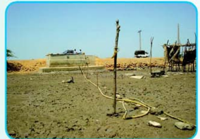
A water storage tank built by the Programme near Keti Bunder Town
