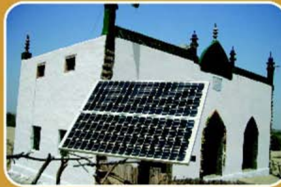
Solar Panel Installed at mosque with PCRET's support
